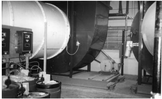
Figure 5. Fan mounted on an inertia base
